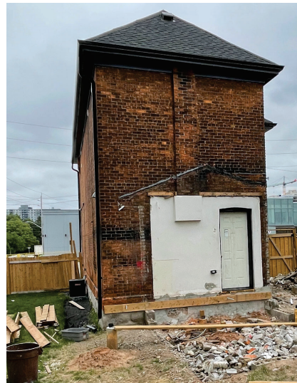
Figure 20. West elevation of the residential building located at 89 Catharine Street North, showing the demolition of the rear portion of the house, which was gabled.
