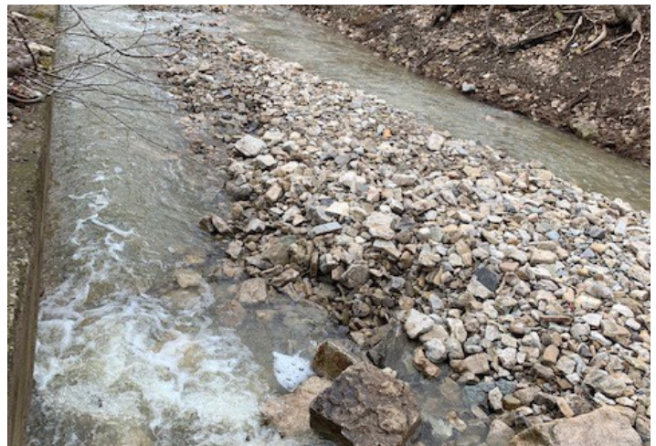
Deposition Site from Erosion in Sydenham Creek. PHOTO City of Hamilton
