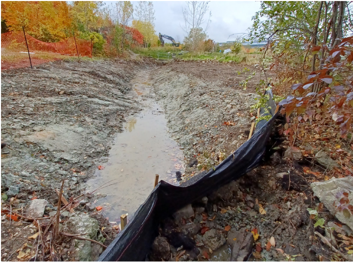
Sediment Control Fencing. PHOTO City of Hamilton
