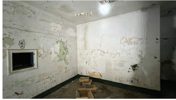
Photo 4: Example of peeling and flaking paint on plaster walls on second floor in the projection room.
