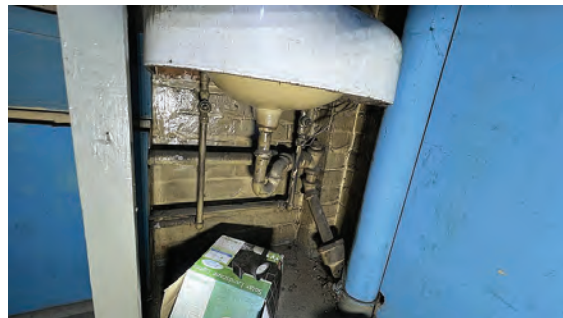
Photo 7: Example of suspected lead-containing pipes and joints.
