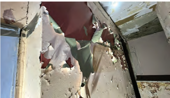
Photo 5: Example of damaged paint on plaster walls on second floor.
