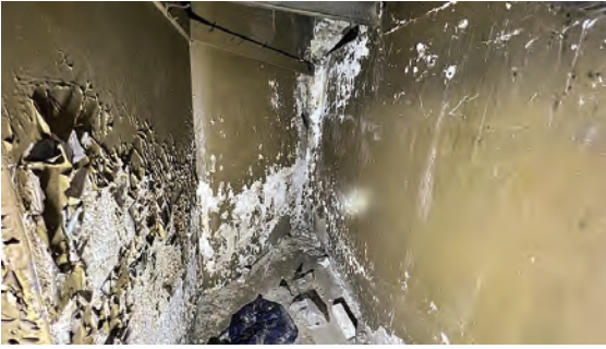
Photo 3: Example of peeling and flaking paint on plaster walls behind stage area.
