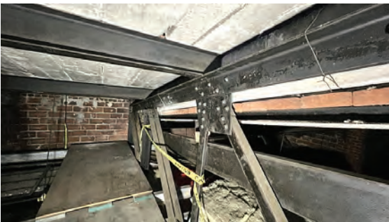
Photo 6: Example of suspected lead-containing primer on structural steel roof framing.
