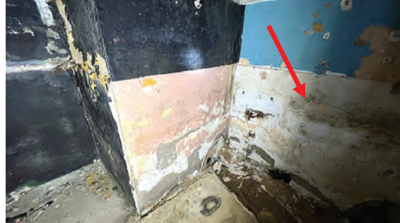
Photo 10: Example of moisture damage on lower walls throughout rooms below stage area.
