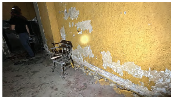
Photo 2: Example of peeling and flaking paint on plaster walls below stage area.
