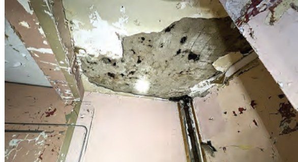
Photo 12: Water-damaged ceiling and mould growth on second floor.
