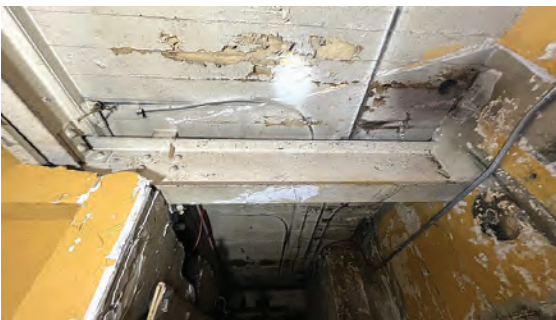
Photo 1: Example of peeling and flaking paint on wood ceilings below stage area.
