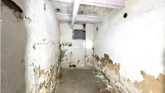
Photo 9: Example of moisture damage and mould growth on lower walls throughout rooms below stage area.
