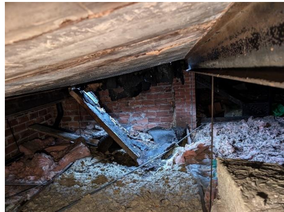
Fig 4: As Fig. 3, in Nov 2024, with failed roof.
