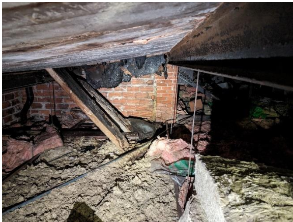
Fig 3: Pier separation, from attic, in Jan 2024.
