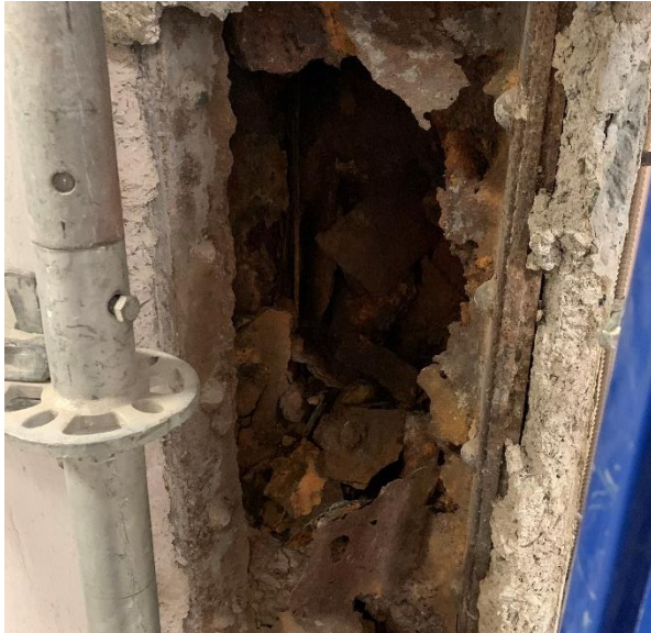
Fig 5: Example of severe concealed corrosion.
