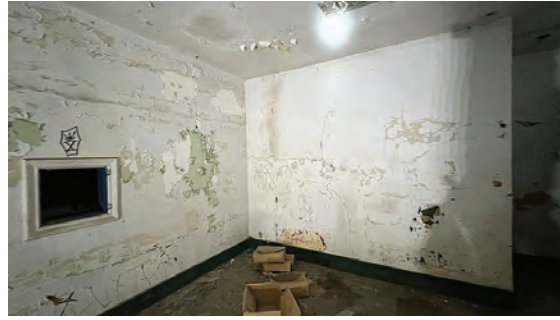
Photo 4: Example of peeling and flaking paint on plaster walls on second floor in the projection room.
