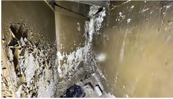
Photo 3: Example of peeling and flaking paint on plaster walls behind stage area.
