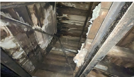
Photo 13: Water damage and mould growth on roofing above catwalk area.
