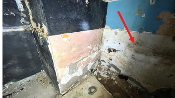
Photo 10: Example of moisture damage on lower walls throughout rooms below stage area.
