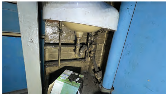
Photo 7: Example of suspected lead-containing pipes and joints.
