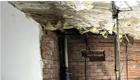
Photo 11: Water damage and mould growth in staircase area leading to projection room.
