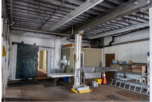
Figure 15: Rear workshop space of 46 Ferguson, with former filled in window openings visible at rear.
