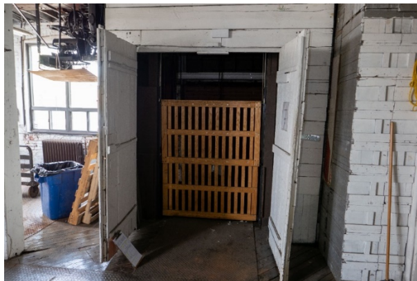
Figure 17: View of the open elevator shaft from the first floor.
