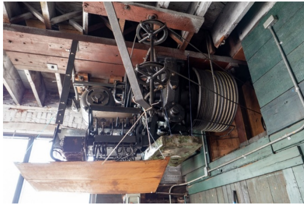
Figure 18: View of the elevator machinery on the west side of the shaft.
