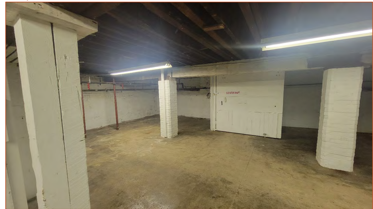
Photo 16. View of the 1909 freight elevator shaft and painted timber beams supported by brick pillars and painted timber posts.
