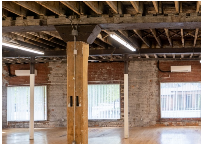
Figure 11: Detail of salvaged wood posts and beams, showing unused joist pockets and tenons.
