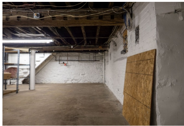
Figure 21: Looking south from the northeast quadrant of the basement at the party wall separating 46 and 48 Ferguson. The former rear foundation wall is at right, with previous window openings visible.
