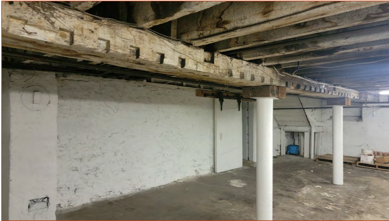
Photo 17. View of the brick foundation walls and timber beams with mortises and timber joists supported by cylindrical metal pillars.
