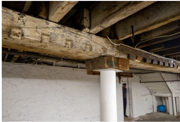
Figure 23: Salvaged wood beams and round posts under the original portion of 48 Ferguson.
