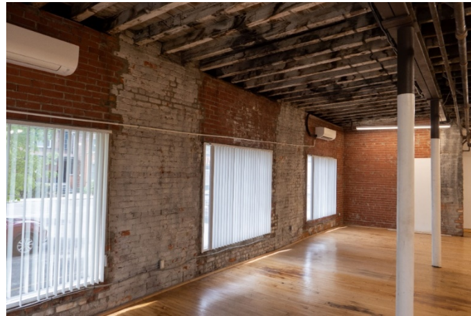
Figure 37: View of Section Z addition interior space, with steel beam and different ceiling structure.
