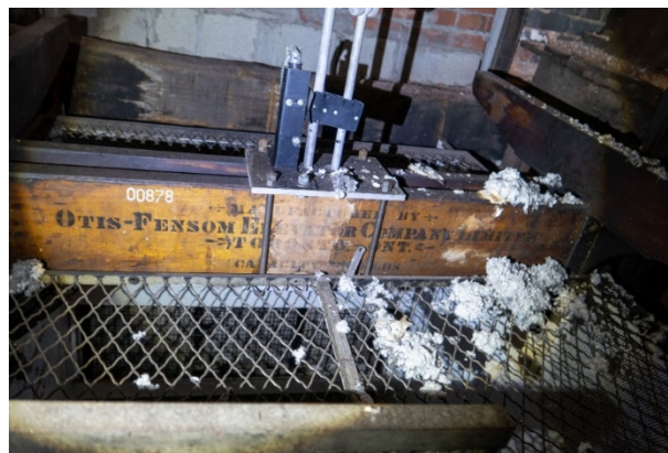
Figure 19: Otis-Fensom top beam of the elevator car.
