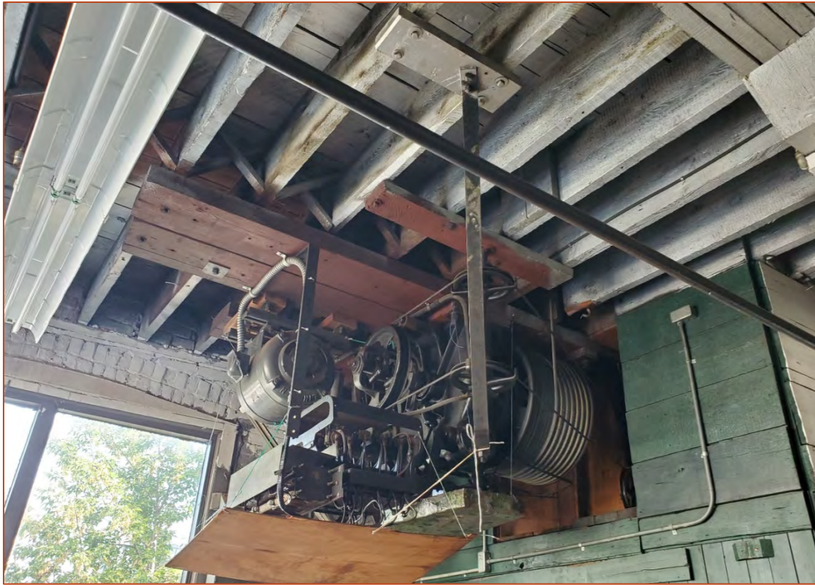
Photo 29. View of the freight elevator motor.
