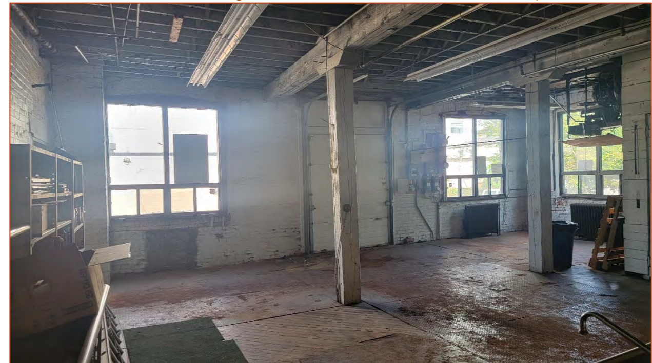
Photo 24. View of the rear workshop area showing wooden timber posts and beams, casement windows, metal grate flooring, and a loading door at centre.
