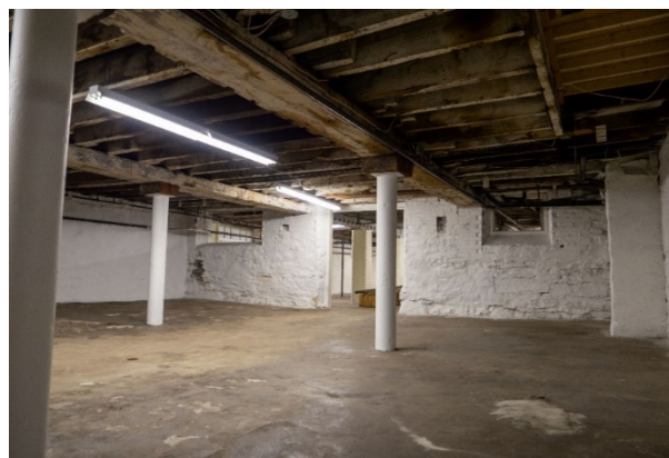
Figure 22: Looking southwest from the southeast quadrant, past the original rear foundation wall and window openings.
