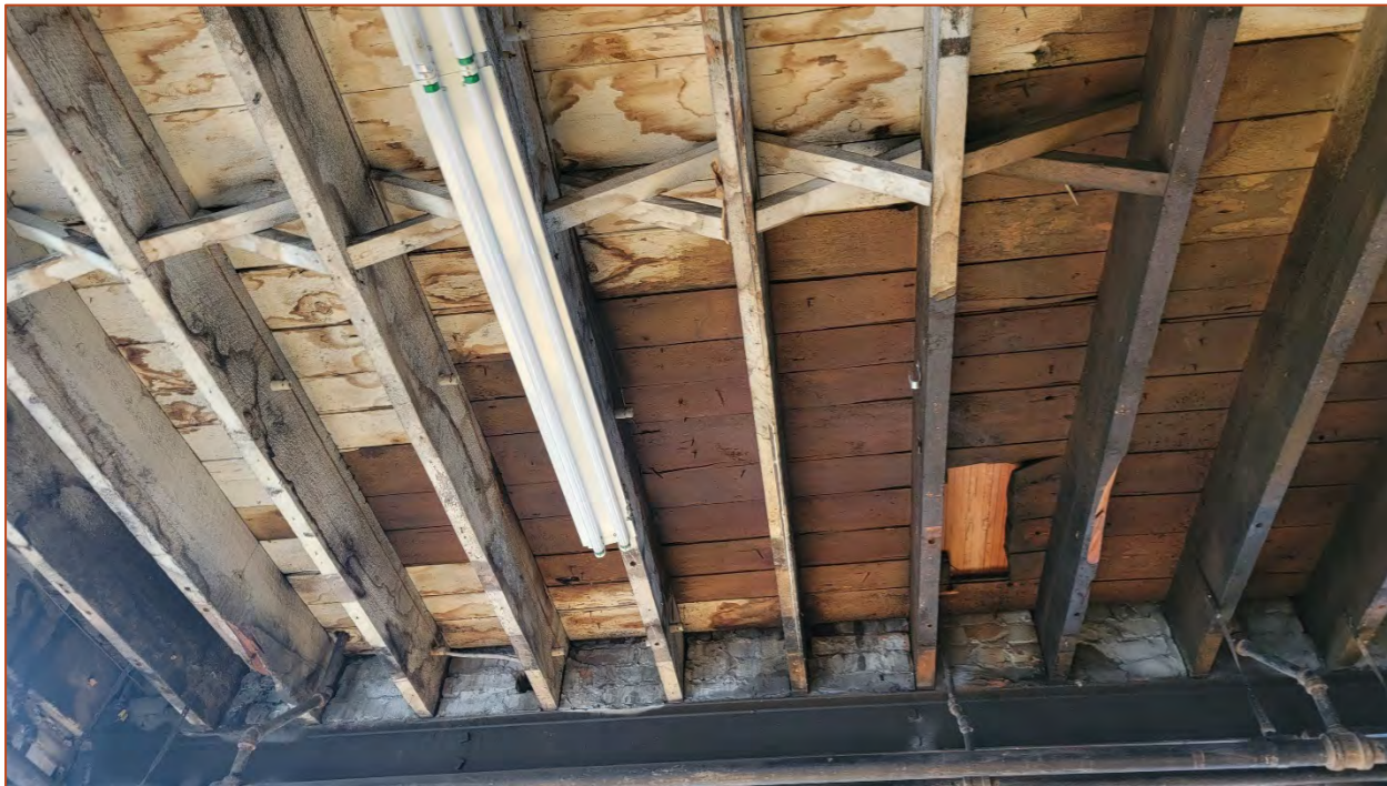
Photo 38. View of the ceiling showing wood boards supported by wooden joists and cross-bracing.
