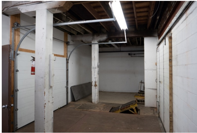
Figure 10: Smaller rooms at rear of 48 Ferguson use smaller posts and built-up beams.
