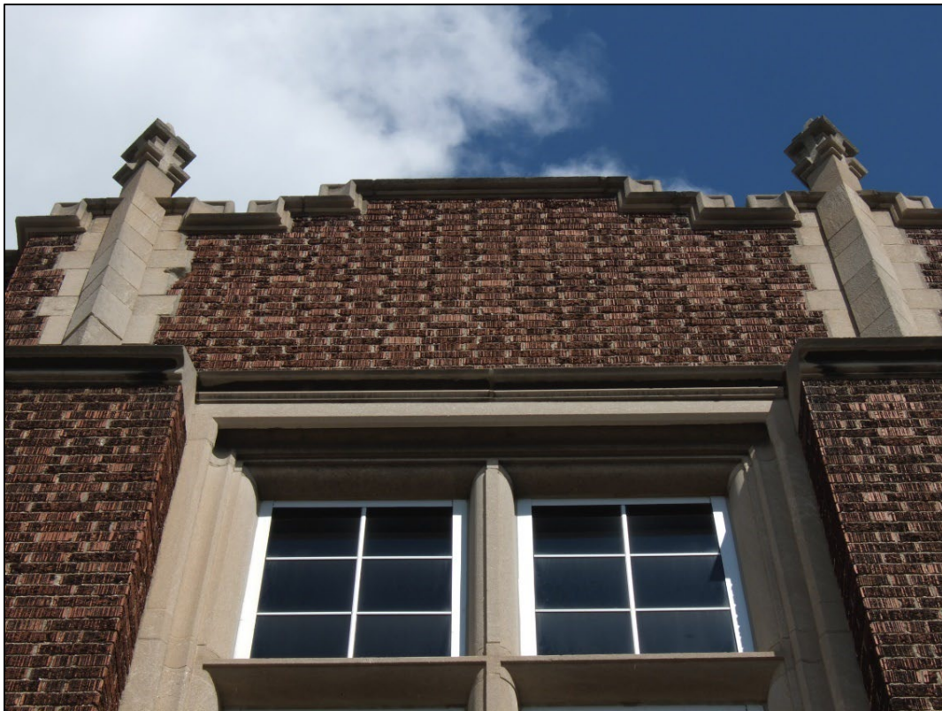
Figure 30: Detail view of parapet over side entrance. City of Hamilton staff July 9, 2014.
