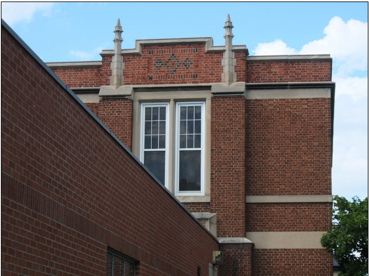
Figure 12: Detail view of decorative elements on the south elevation of the 1921 Manual Arts Building. City of Hamilton staff, July 9, 2014.
