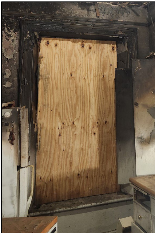
Figure 5: View from interior of one window to be replaced, due to damage from the fire.
