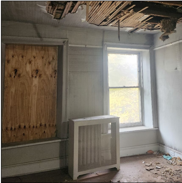
Figure 4: View from interior of one window to be replaced and one to be restored.
