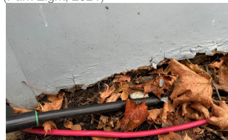
Painted particle wood siding with matching painted corner caps being rotted at grade (Park Eight, 2024)
