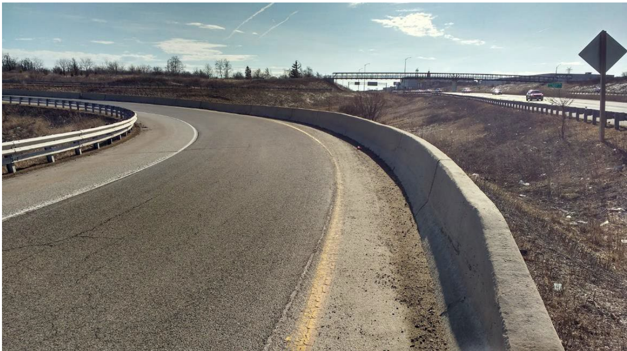
Figure 25: Interchange Ramp Issues, including Trumpet Ramps
