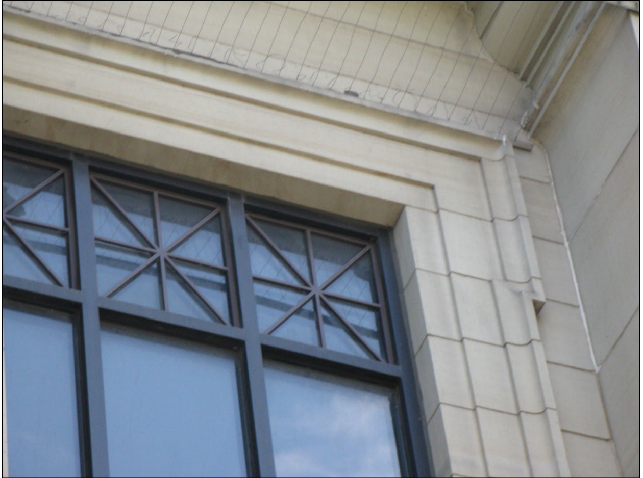
Image 6: Close up of multi-pane metal windows with decorative metal Roman lattice window grillwork (July 10, 2012)
