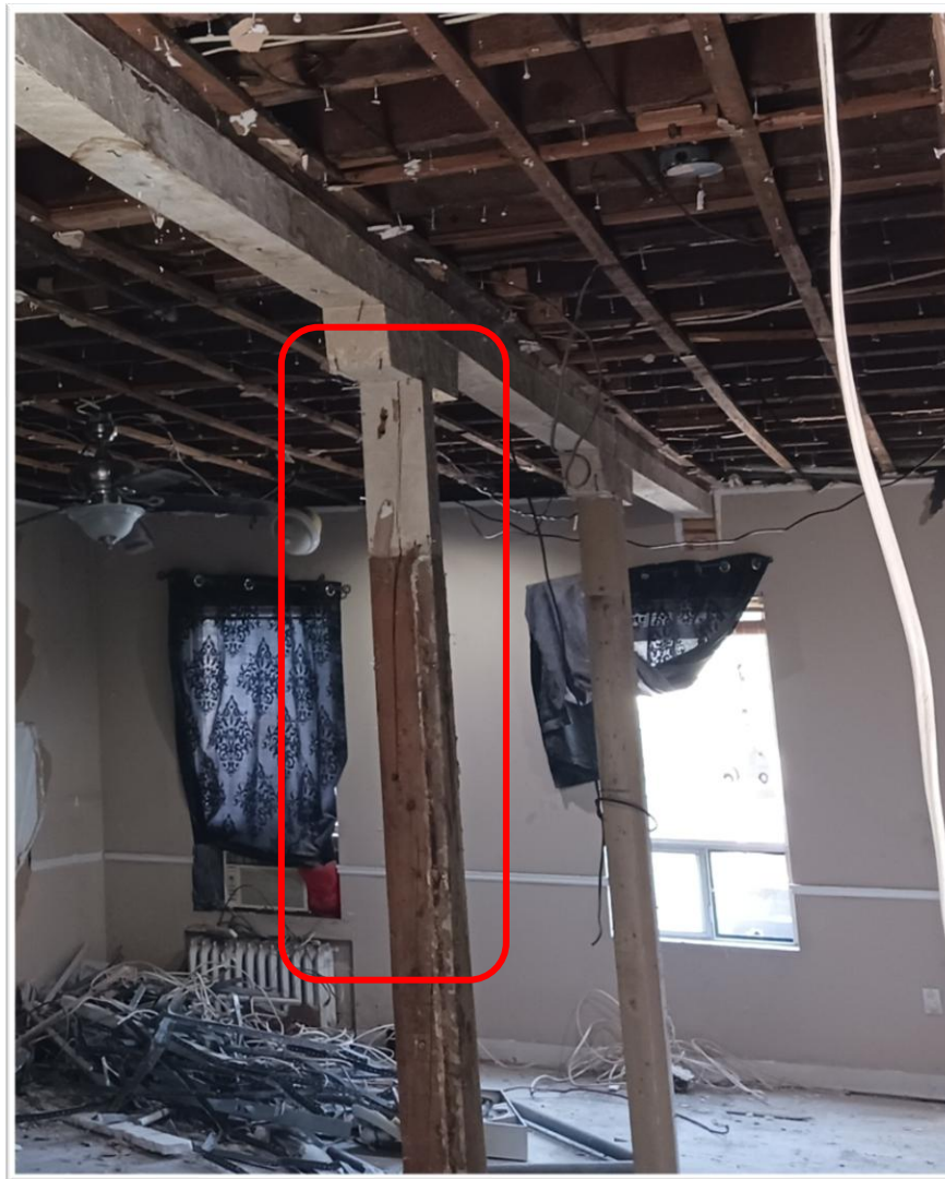
Figure 11: Cracked Structural Column
