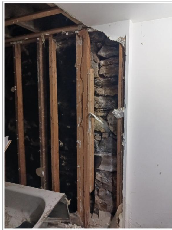
Figure 3: Damaged Foundation wall
