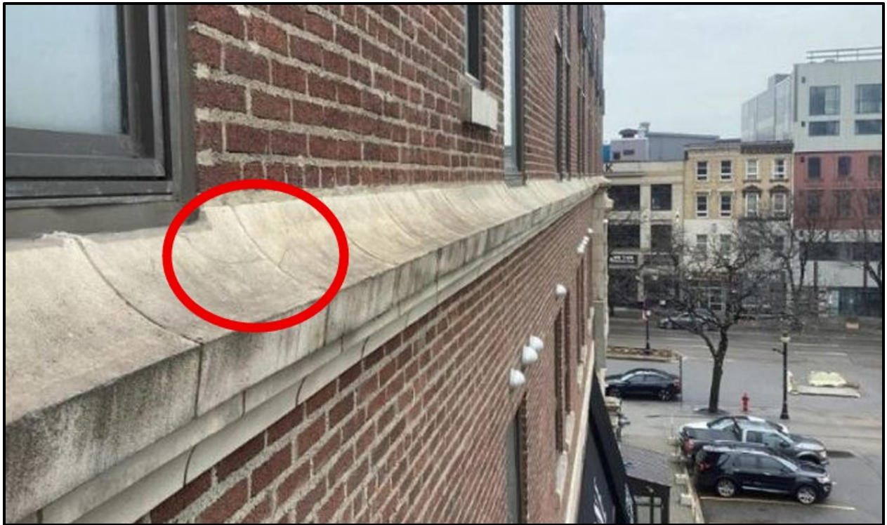
Figure 5: Close up example of a cracked cast stone in need of repair along the east elevation (Proponent Submission, 2026)
