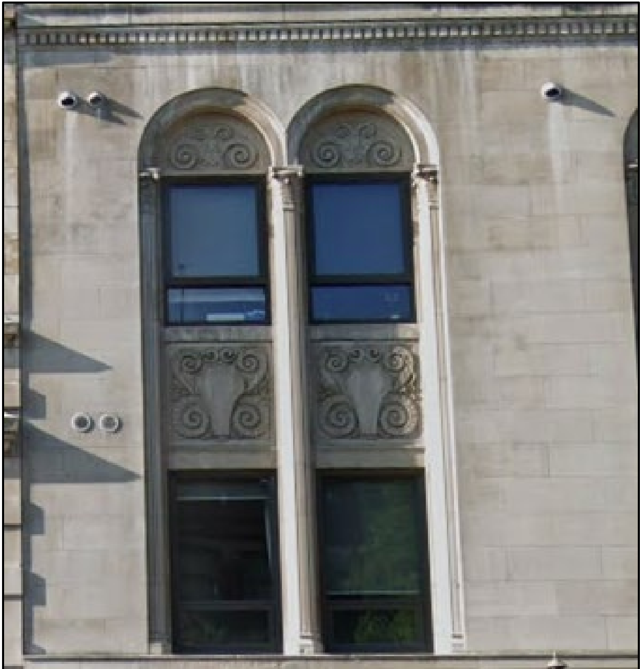
Figure 6: Close up example of cast stone to be cleaned along the north elevation (Google Earth, 2021)
