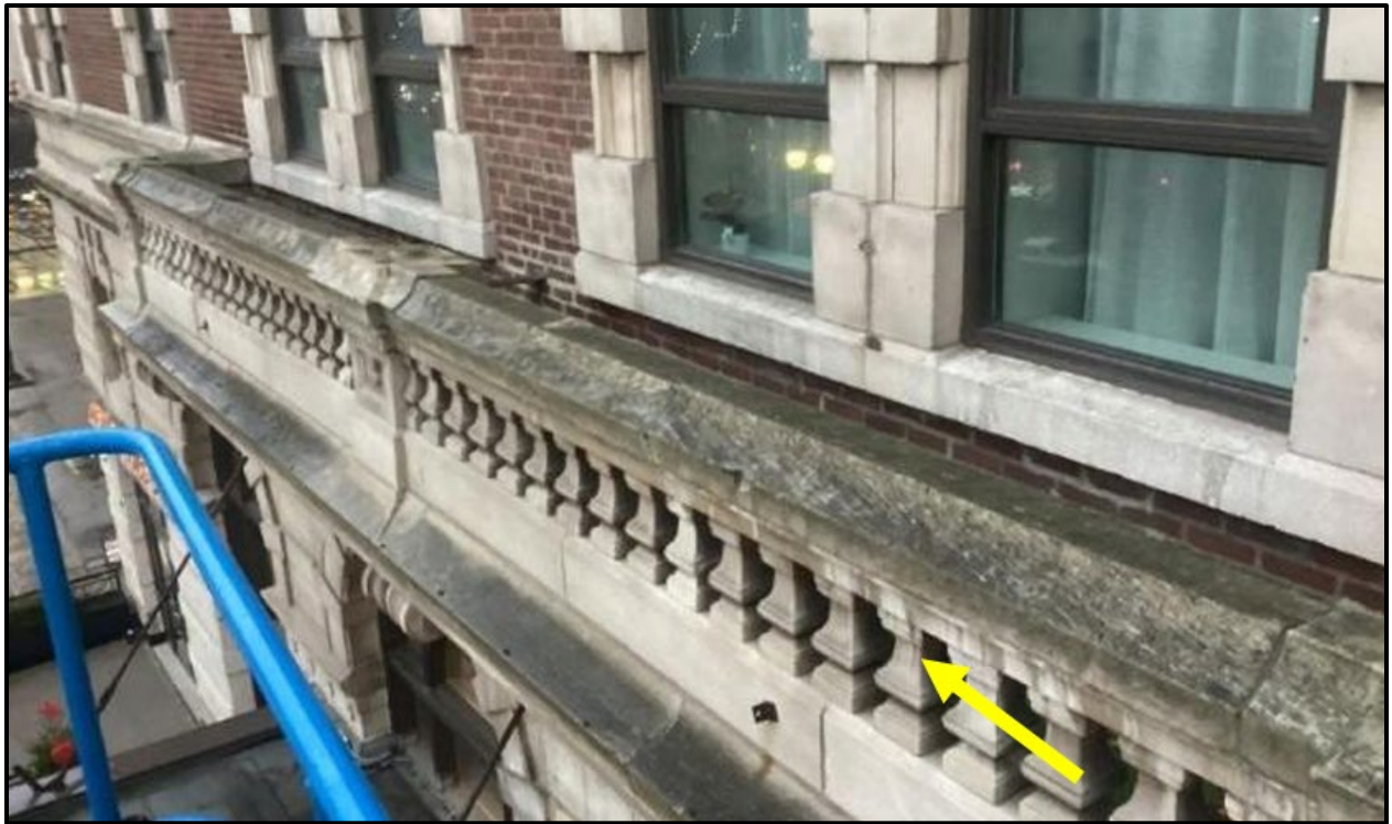
Figure 6: Close up example of cast stone to be cleaned along the north elevation (Proponent Submission, 2026)
