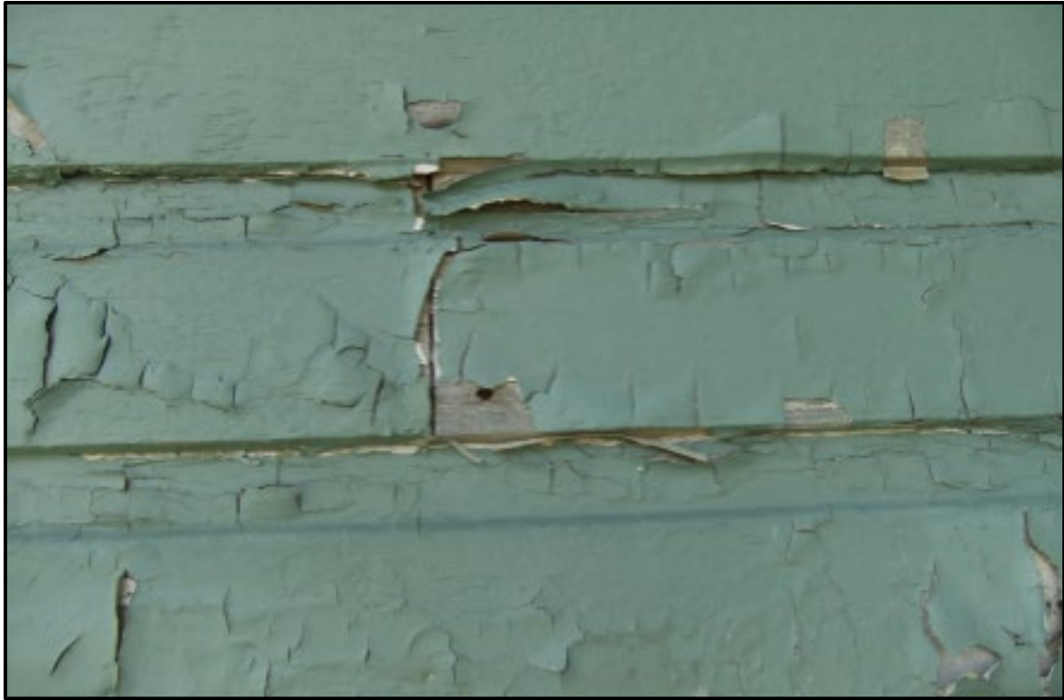
Figure 4: Close up of the deteriorated siding to be replaced, including peeling paint and rotting wood (Site Visit, 2024)
