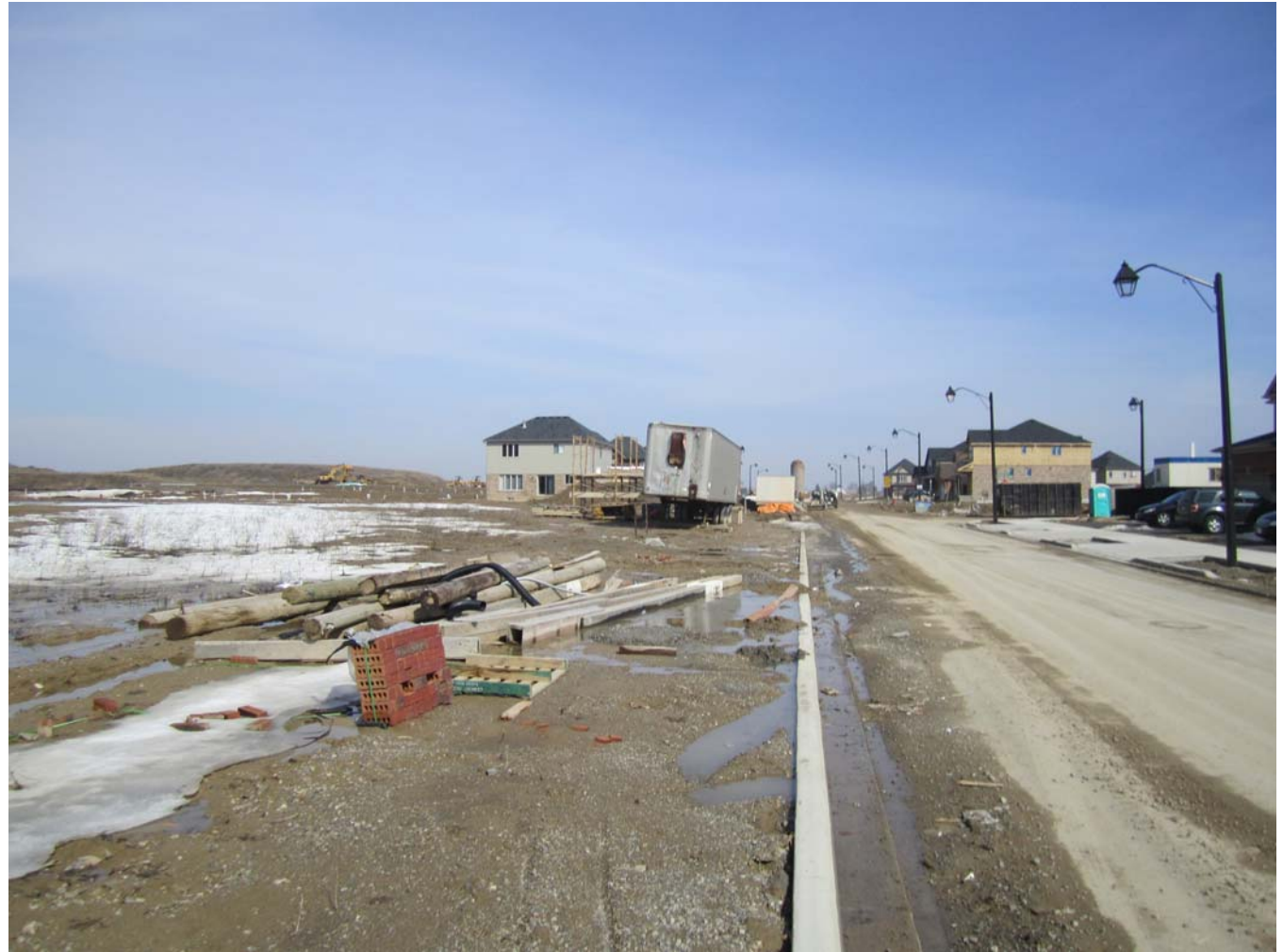
Photo 2 - View to the North of the Subject Lands along Royal Winter Drive
