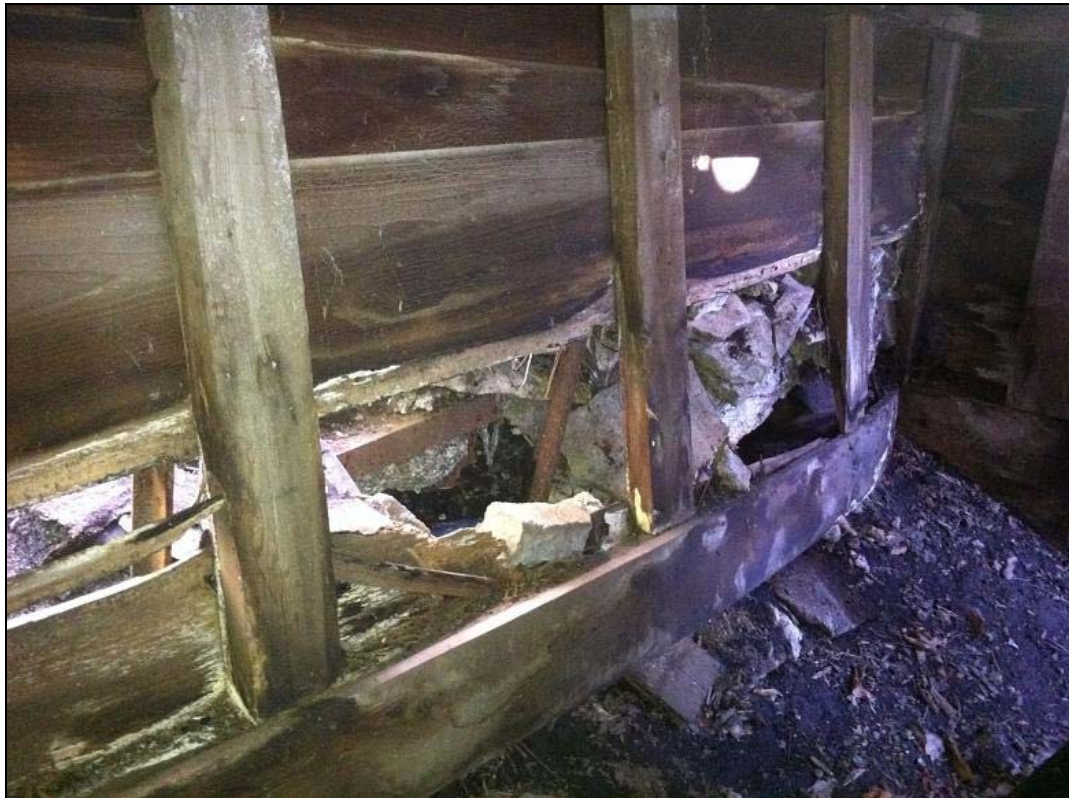
Deteriorated lower walls and lack of foundation/footings in existing garage.
