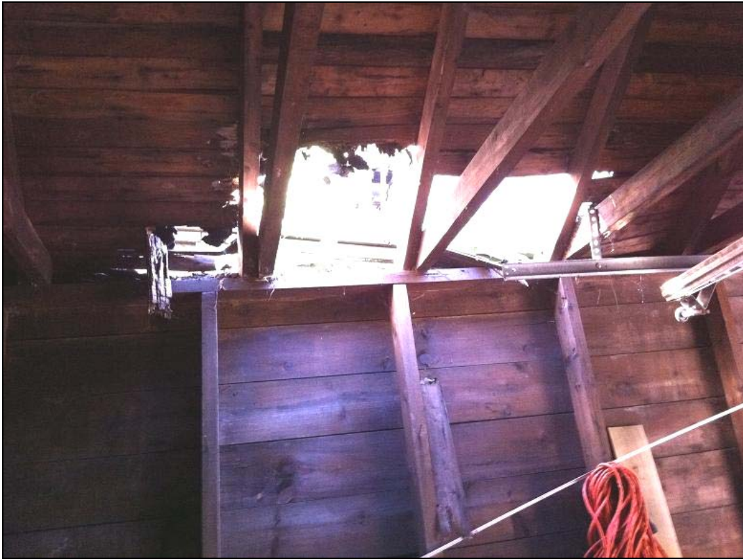
Deteriorated roof on existing garage.
