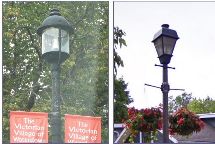
Figure 25 - Traditional Style Luminaires
