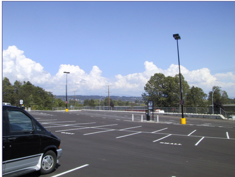
Figure 56 - Recommended Parking Lot Lighting
