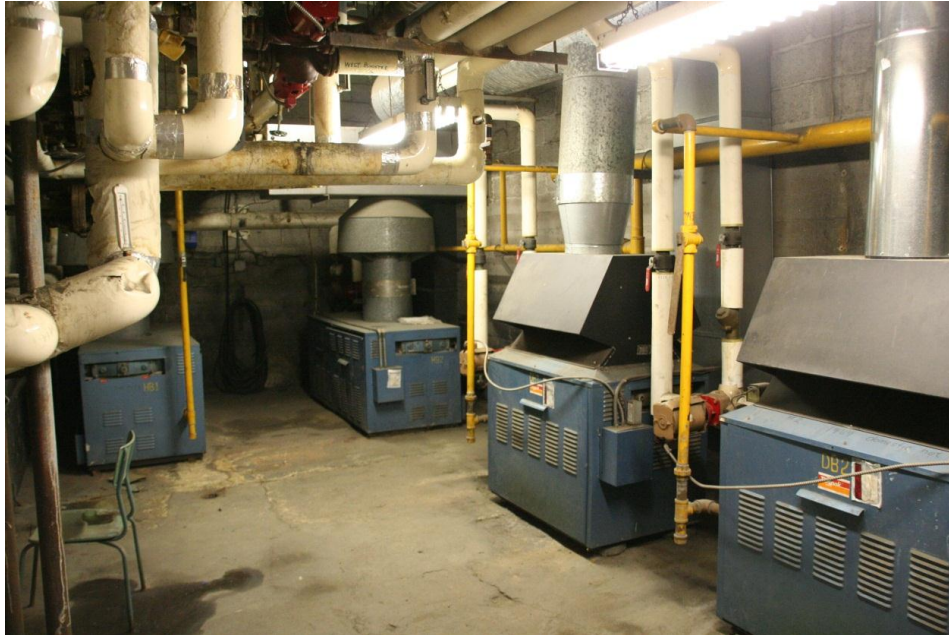
Figure 28: Furnace room containing modern furnaces. The exterior chimney is outside the wall at the furthest furnace.
