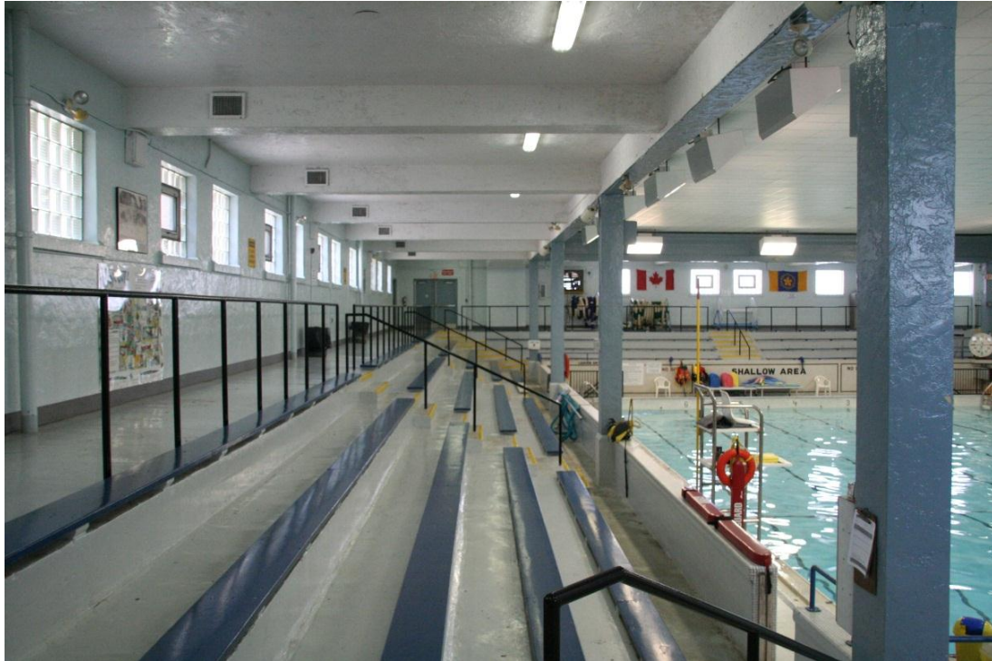
Figure 33: Bleachers on west side showing window patterns, roof posts and beams and 2004 emergency escape door
